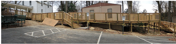
Tallwood ramp built by Mason Facilities Management for Americans with Disabilities Act compliance is nearing completion as shown in panoramic view
